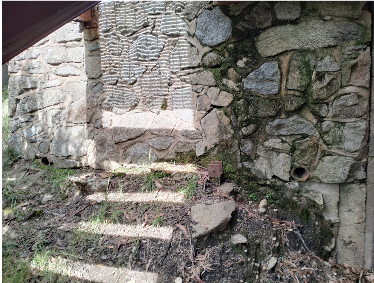
KOSCIUSZKO THREDBO PTY LTD PROPOSED DEMOLITION & REDEVELOPMENT - SONNBLICK LODGE – 10 BOBUCK LANE, THREDBO, NSW SITE PHOTOGRAPH – RW3
